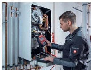
Testing of gas pressure regulators
