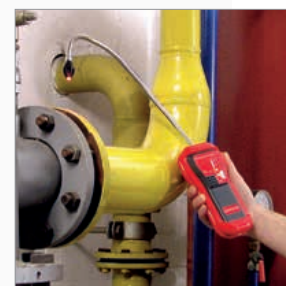
Finds leaks easily
